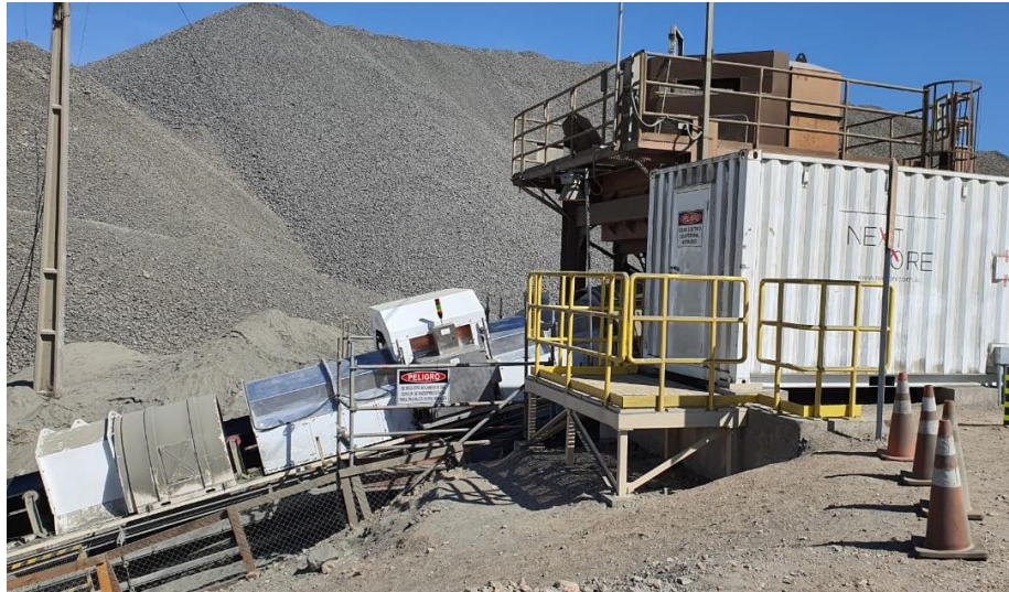
Figure 2 MRA installed con crusher discharge conveyer CV-02
