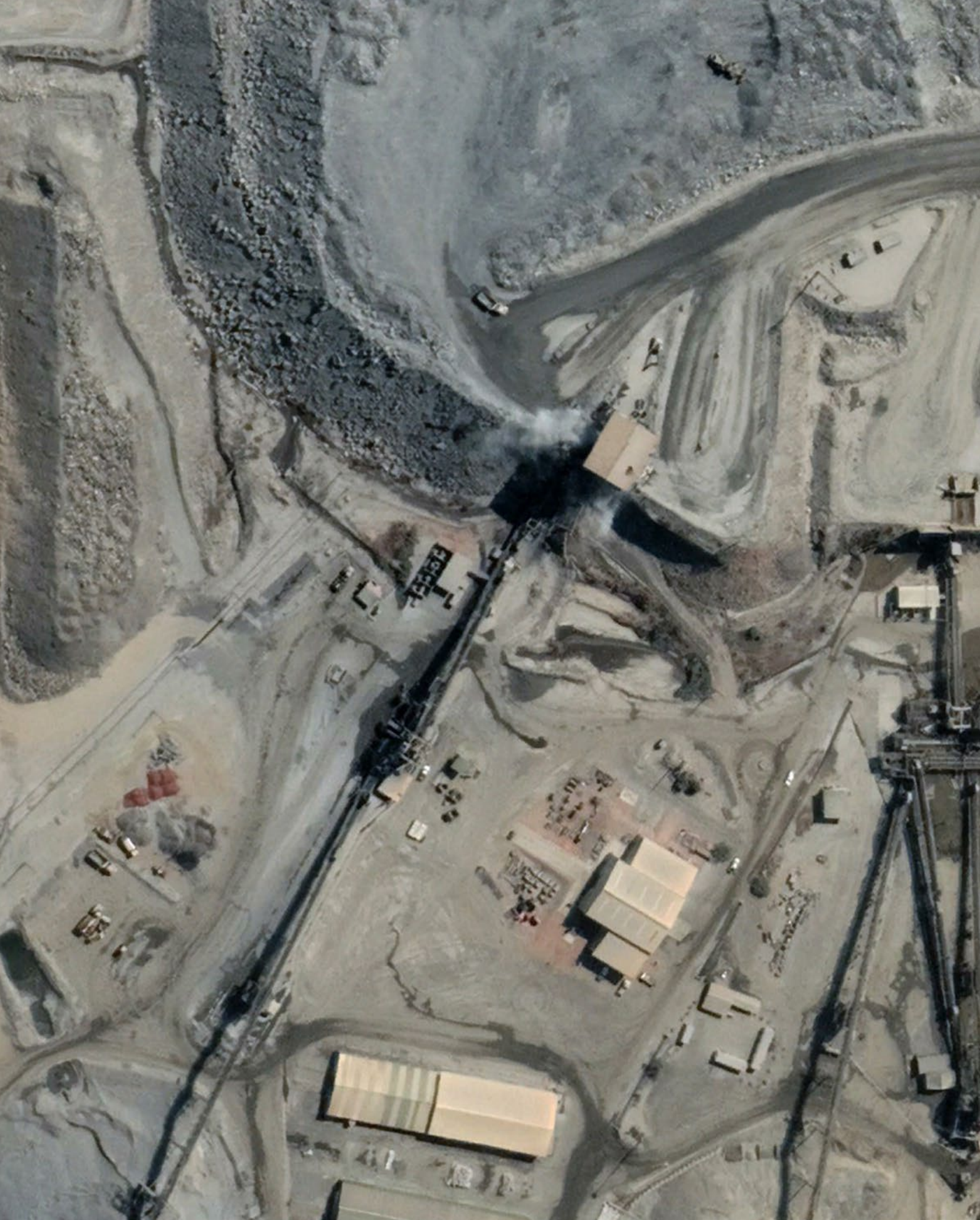
Figure 3 - Satellite image of Kansashi sulphide primary crushing circuit in August 2021 (left) and June 2022 (right), after installation of BOS equipment.
